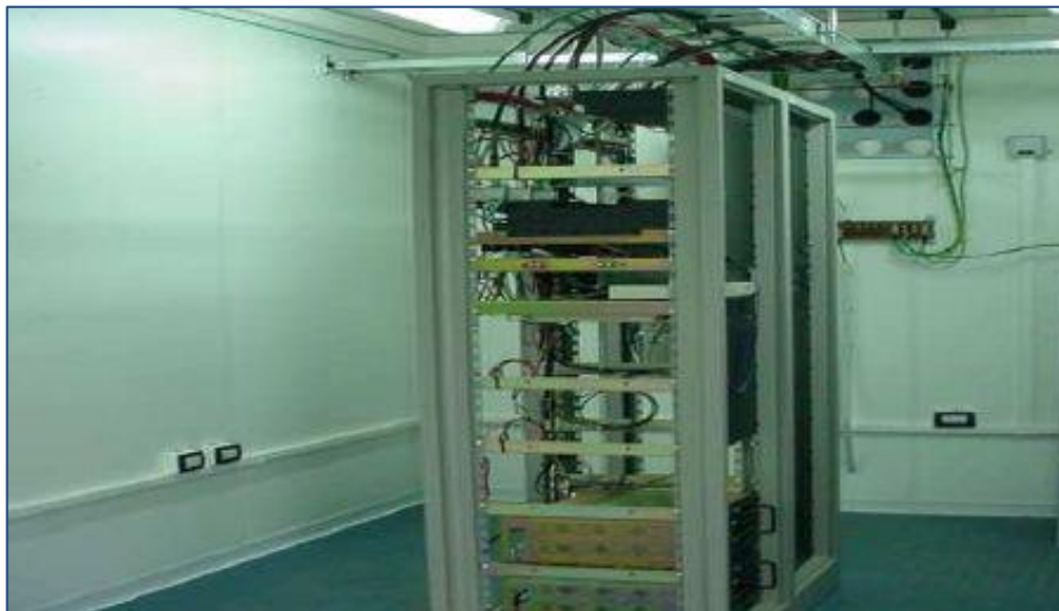
Figura 23 - Racks en Shelter
