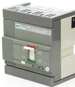
Figura 94: Interruptor diferencial principal
